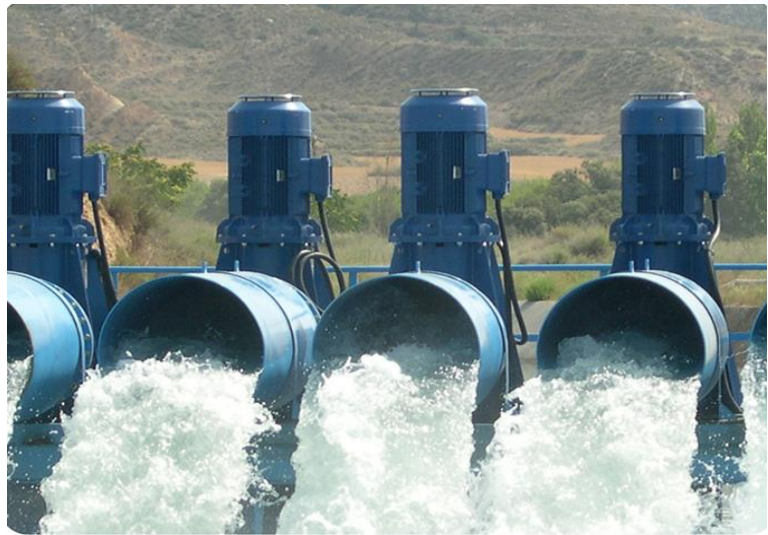
SPI OPERATES UP TO 500 HP SURFACE PUMPS WITH SOLAR
