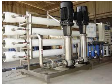
S : Skid based plant
