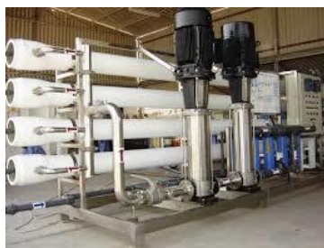
Skid mounted plant
